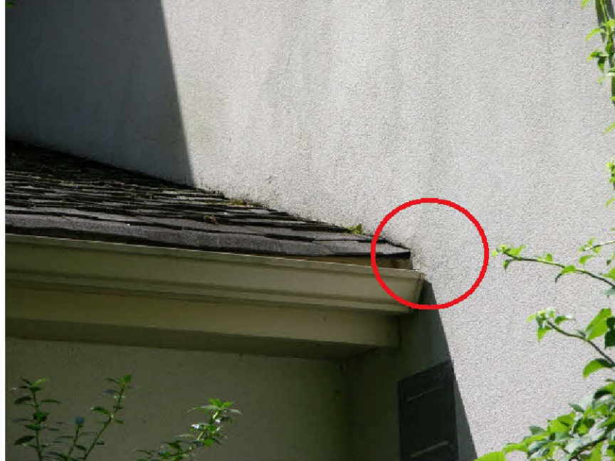
MISSING ROOF-WALL DIVERTER FLASHING. NOTE CRACK IN STUCCO.
