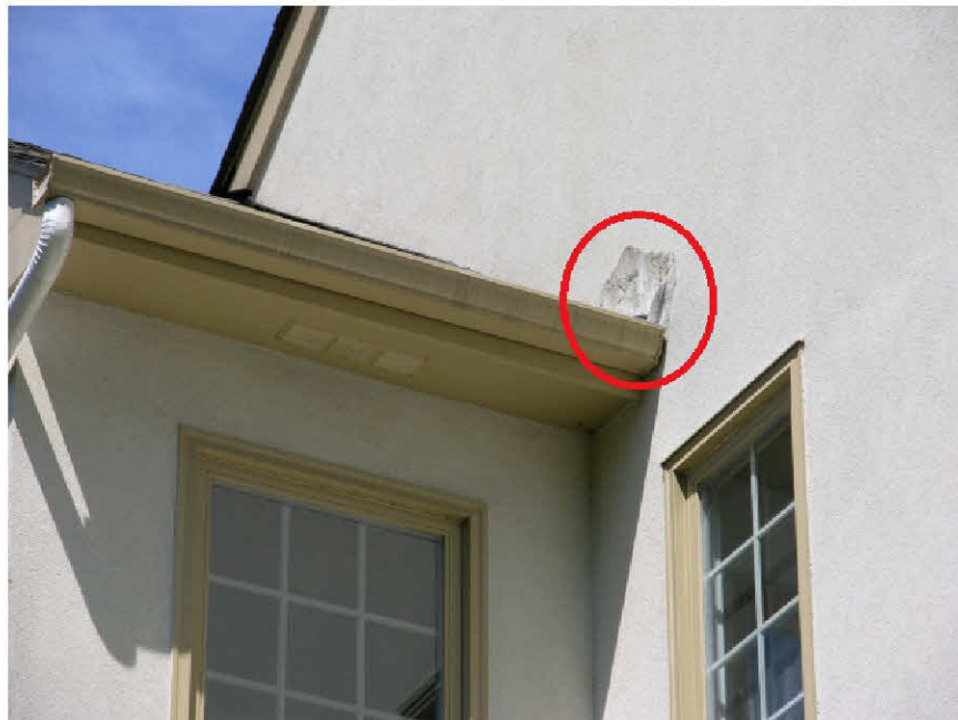
IMPROPER AND UNSIGHTLY INSTALLATION OF ROOF-WALL DIVERTER FLASHING POSTAFTER CONSTRUCTION.
