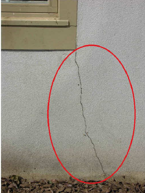
OPEN CRACK IN STUCCO. PORTAL FOR WATER INTRUSION.
