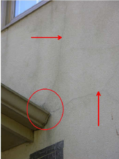
CRACKING PATTERN IN STUCCO.
