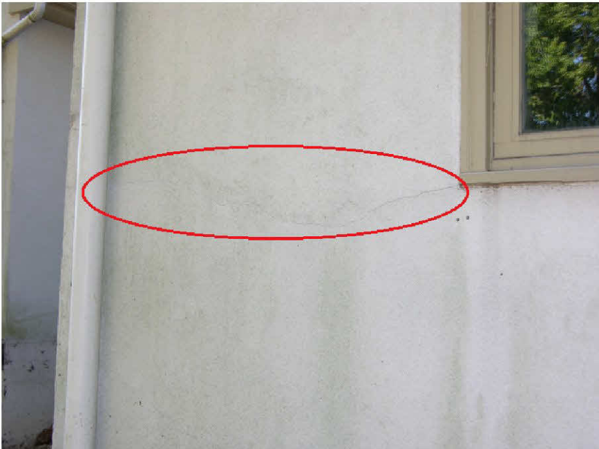
CLOSE-UP OF CRACKING PATTERN FROM WINDOWS TO EDGE OF STRUCTURE.
