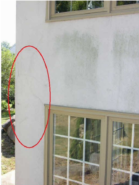
REAR ELEVATION - LEFT QUADRANT STUCCO CRACKING.
