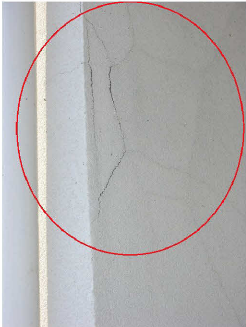
DETAIL OF STUCCO CRACKING AND SPALLING.
